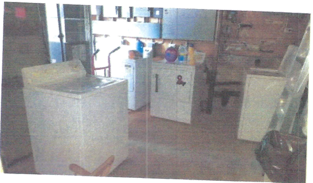
View: Utility and furnace room on the southwest side of the site building
