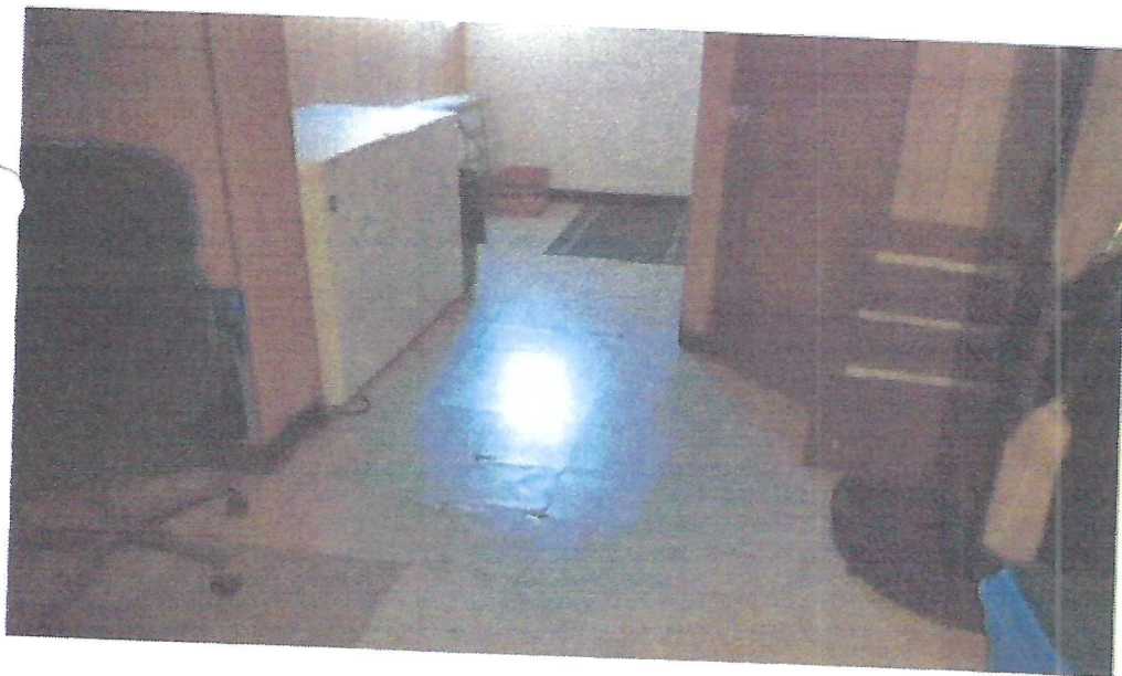
View: Broken floor tiles located in the central portion of the basement
