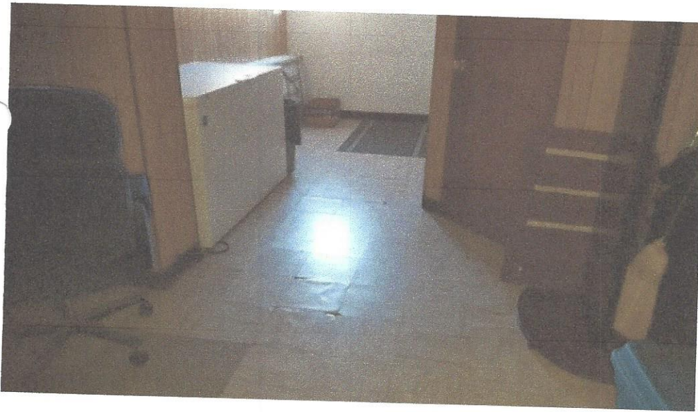
View: Broken floor tiles located in the central portion of the basement
