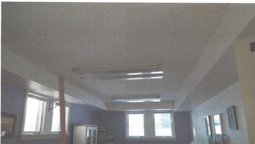
View: Typical ceiling tile located in the ground floor
