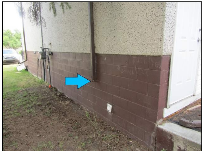
Should discharge 6 feet from building
