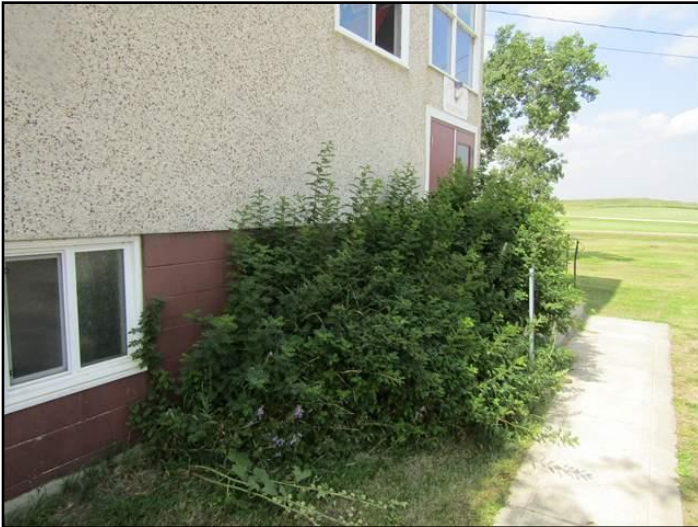
Trees or shrubs too close to building
