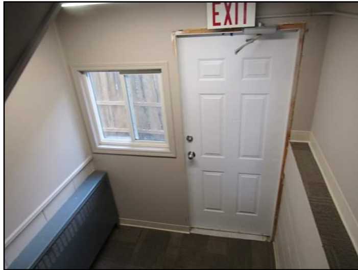
Rear entrance door/mechanical damage
