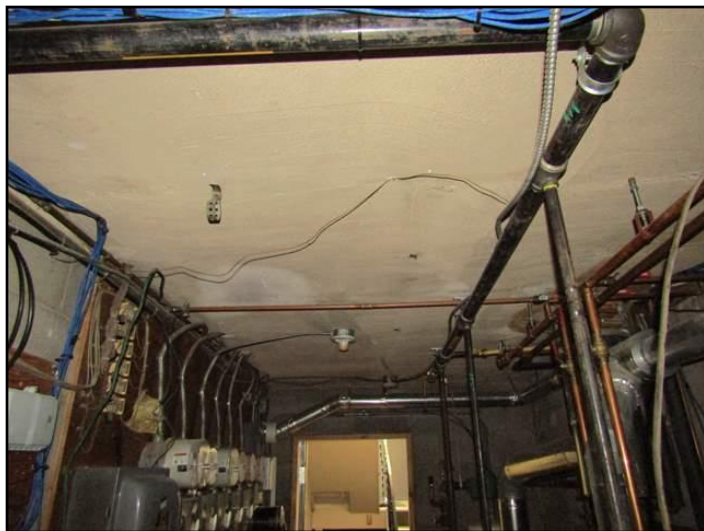
Possible asbestos ceiling board
