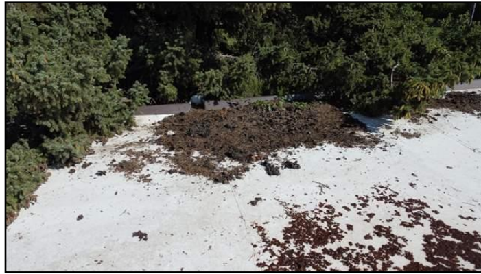
Debris on roof
