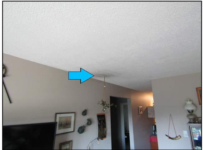
Marks on ceiling (unit 6)
