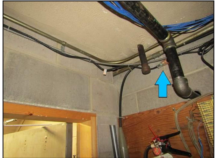
Extension cord used as permanent wiring
