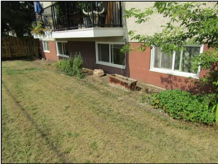
Improper slope or drainage
