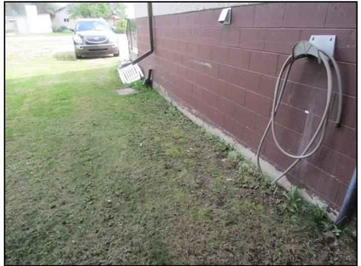
Improper slope or drainage
