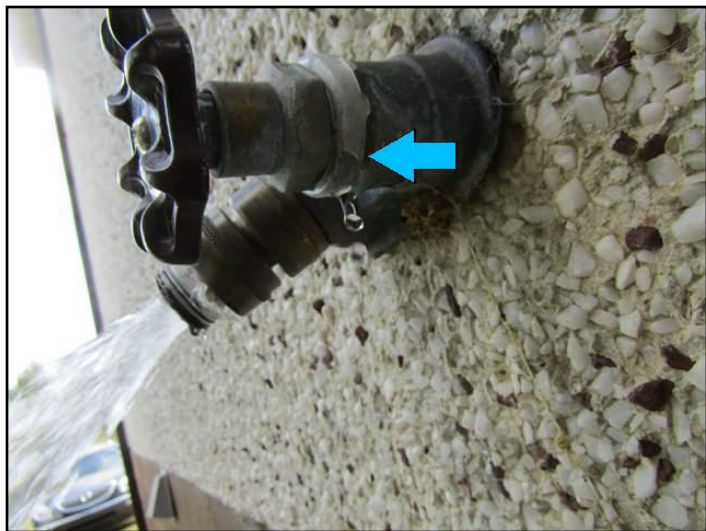
Leak or drip
