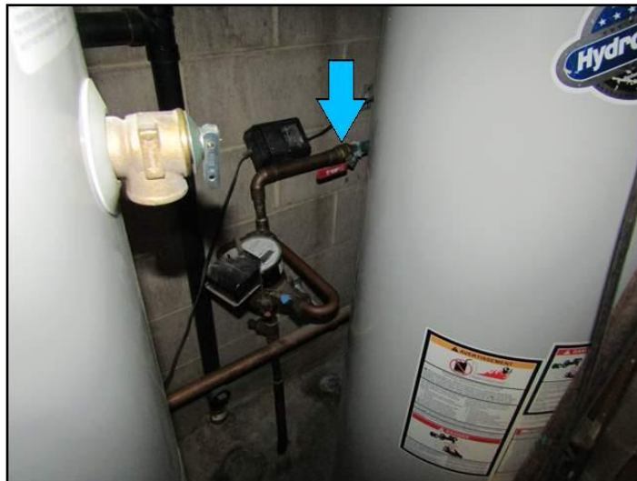
Near water heater
