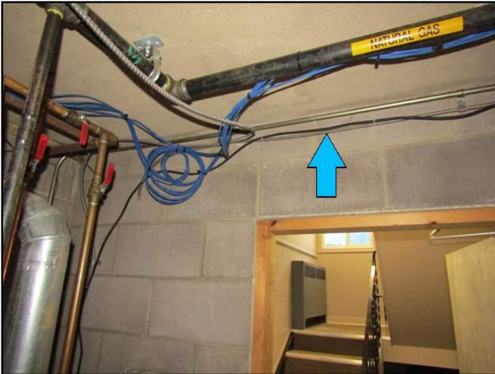
Extension cord used as permanent wiring
