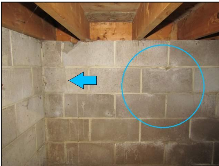
Crack on block as well as Step crack
