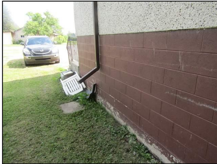
Should discharge 6 feet from building
