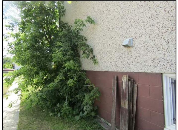
Trees or shrubs too close to building
