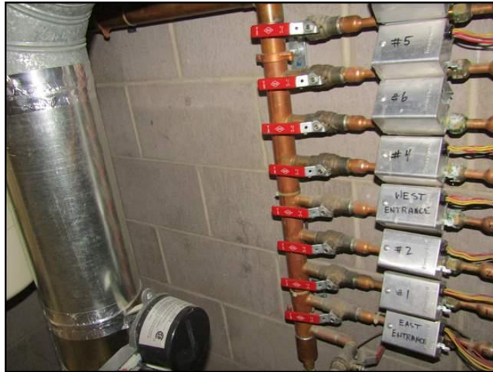
valves for units 2 and 5 should be replaced
