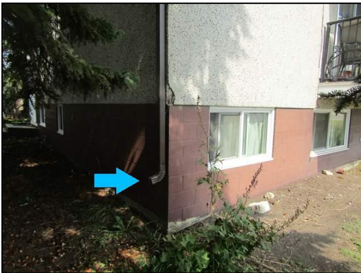
Should discharge 6 feet from building
