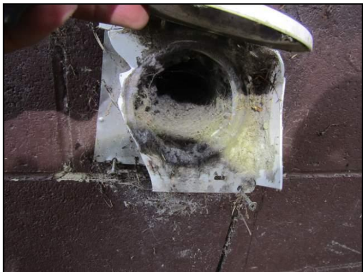
Dryer vent obstructed
