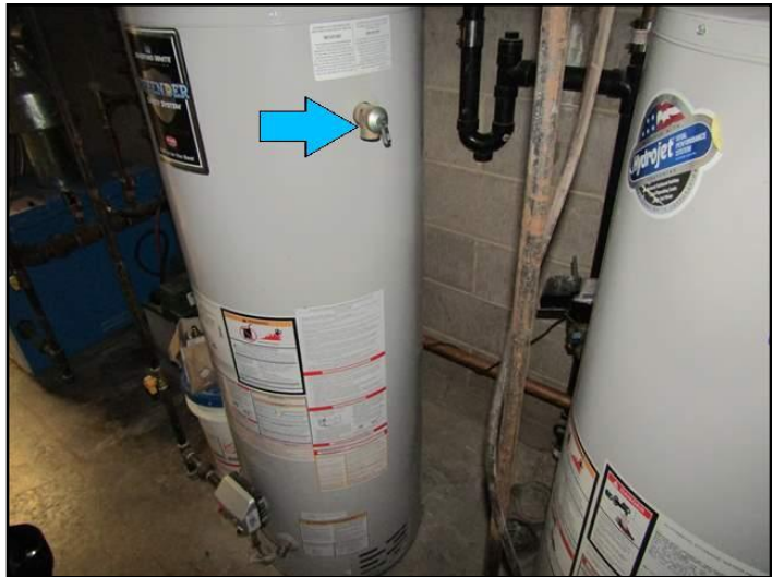
Discharge tube missing
