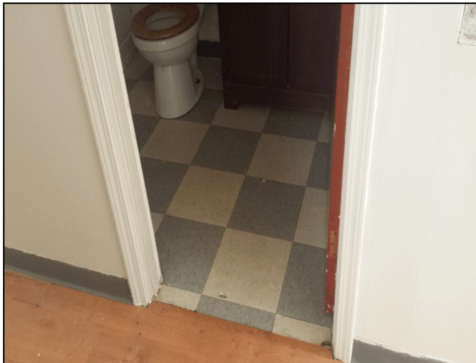
Photograph 7: Looking at the wood laminate flooring overlying vinyl tile noted in one of the renal units (March 5, 2015).
