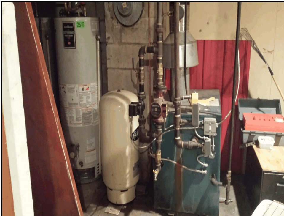
Photograph 11: Showing the boiler and hot water tanks in the utility room of the building, with concrete floors, unpainted concrete block and painted drywall finishes (March 5, 2015).
