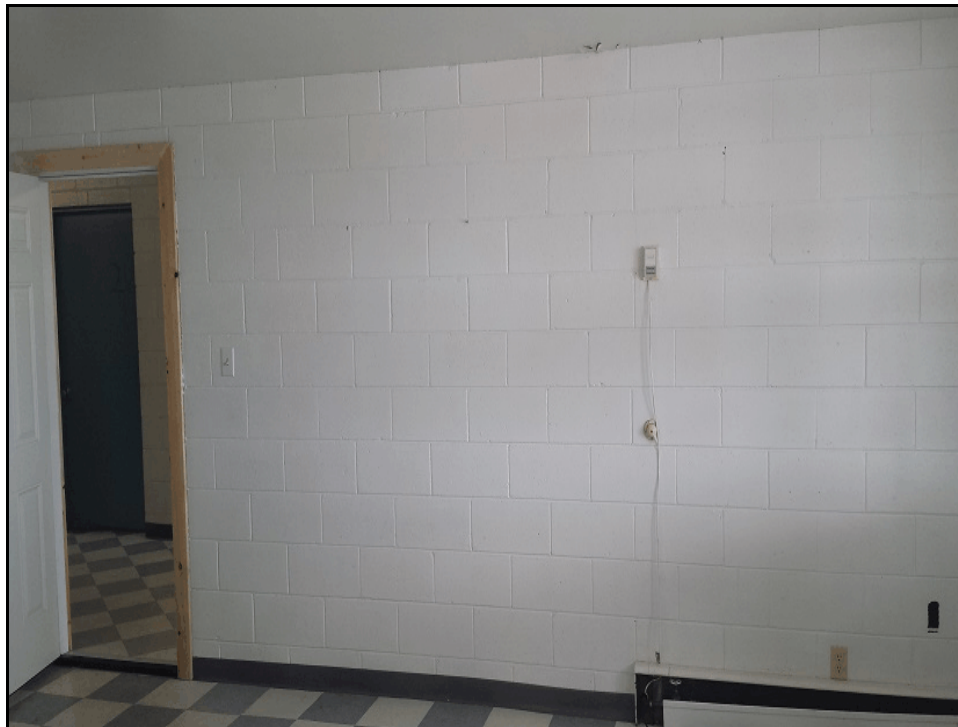
Photograph 6: Showing a mercury thermostat, baseboard heater and painted concrete block finishes in one of the rental units (March 5, 2015).
