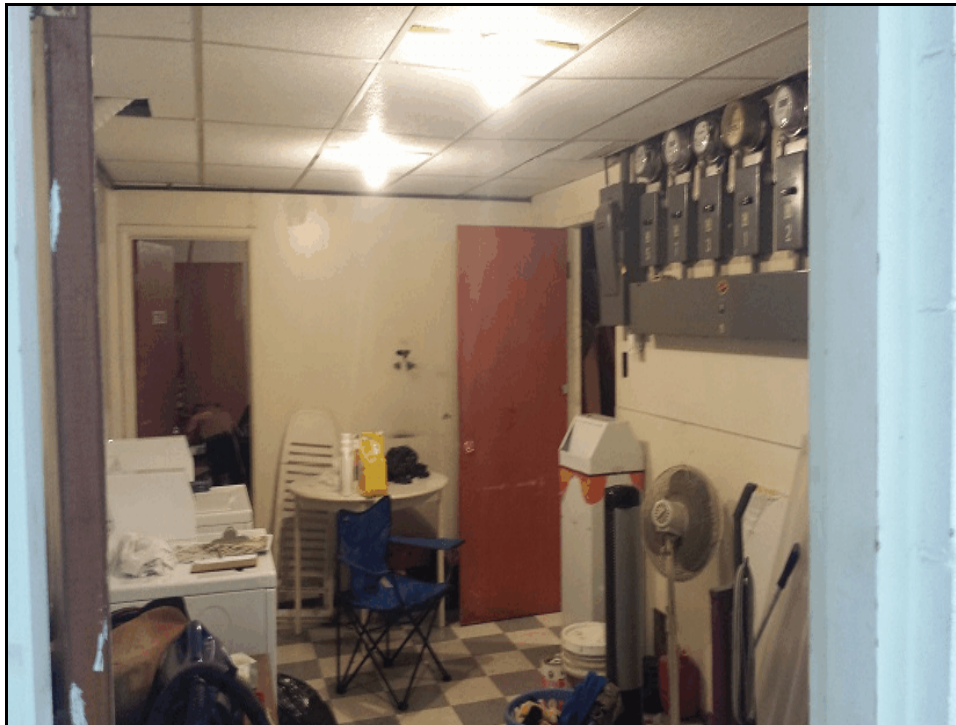
Photograph 9: Facing the laundry room, showing painted drywall and drop-tile ceiling finishes, vinyl flooring, electric panel meters and controls, laundry machines and miscellaneous storage (March 5, 2015).
