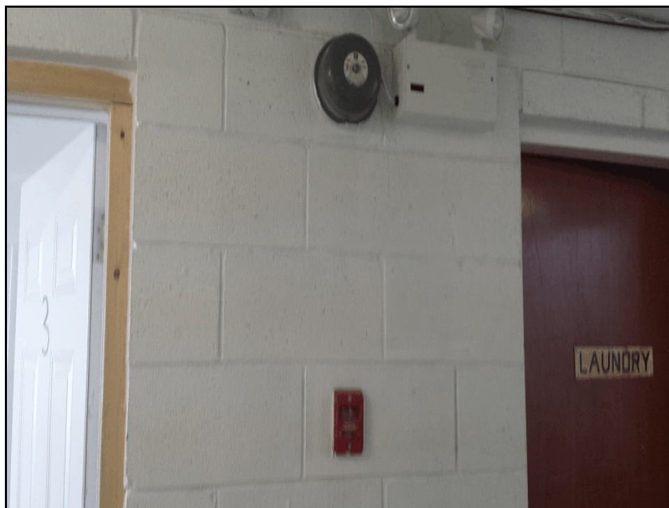
Photograph 8: A close-up of the fire alarm and emergency light system in the hallway of the building (March 5, 2015).
