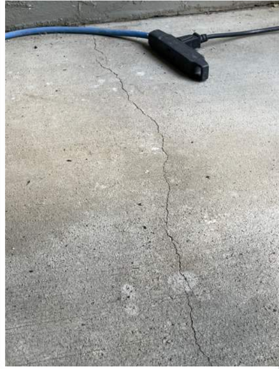
Cracking observed on the concrete. RCMD filling cracks and sealing floor with paint or epoxy
