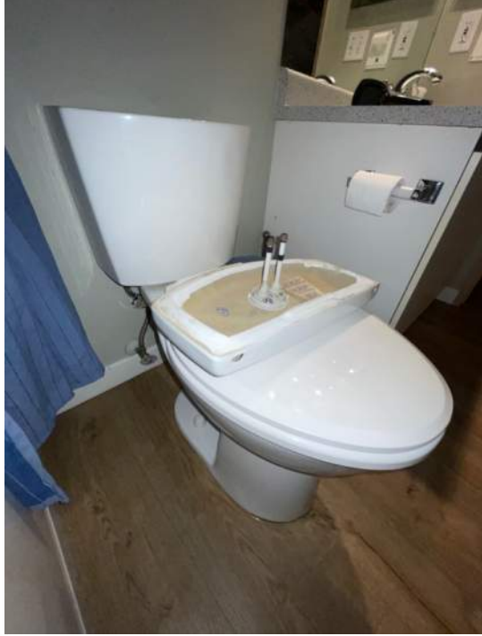
Toilet base thermal scan example.
