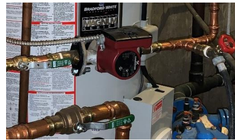
Figure 6 - DHW Recirculation Pump
