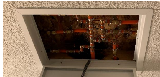
Figure 4 - 2nd Floor Ceiling
