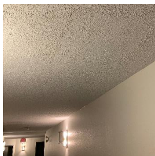
Figure 2 - 2nd Floor Leaks Location
