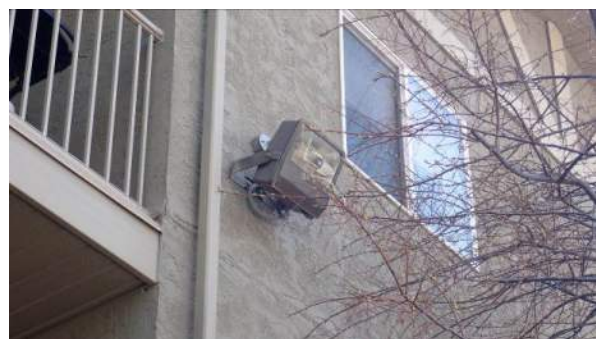
Exterior Lighting - Common
