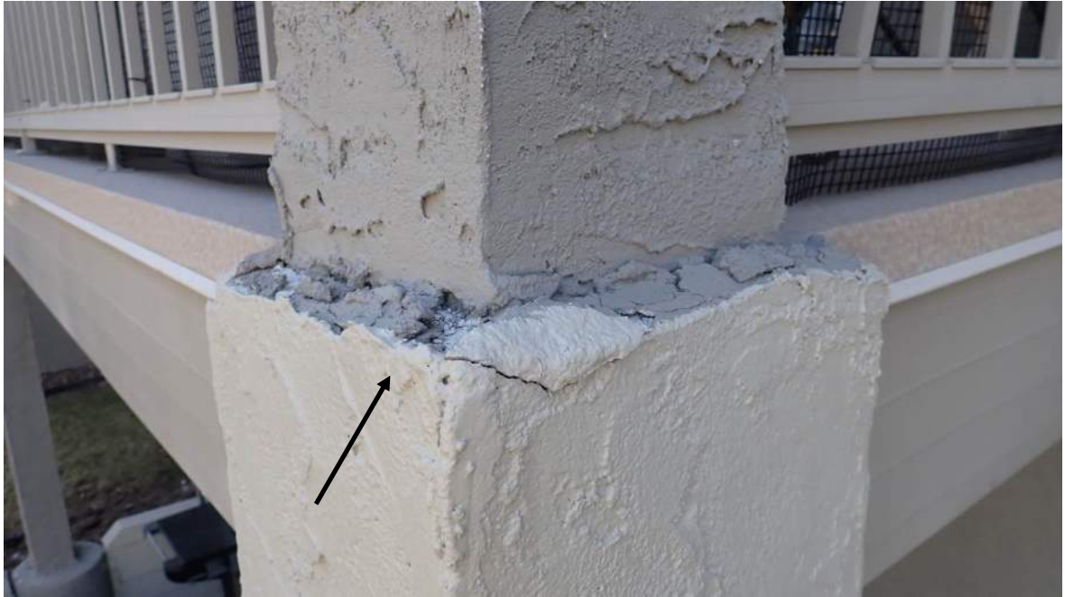
Photo 5 Localized Stucco Damage at Balcony Column
