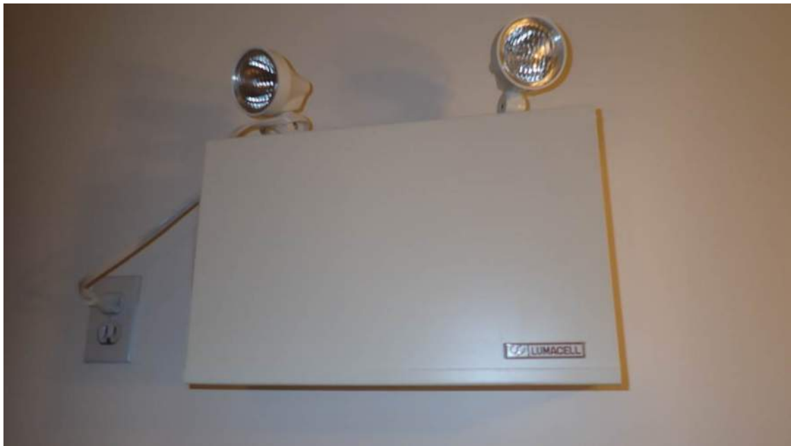
Photo 2 Typical Emergency Light with Battery Pack
