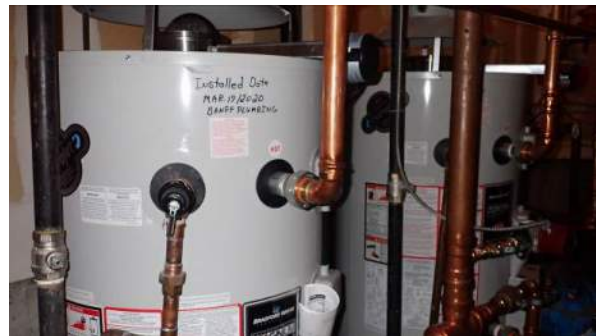
Domestic Hot Water Tanks
