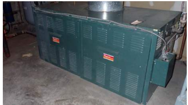
Natural Gas Boiler System
