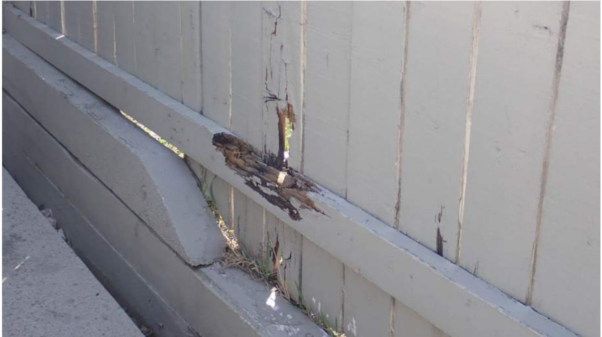
Photo 9 Deterioration of Garbage Enclosure
