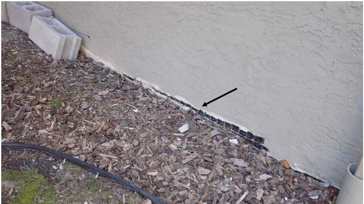
Photo 4 Localized Stucco Damage on North Elevation
