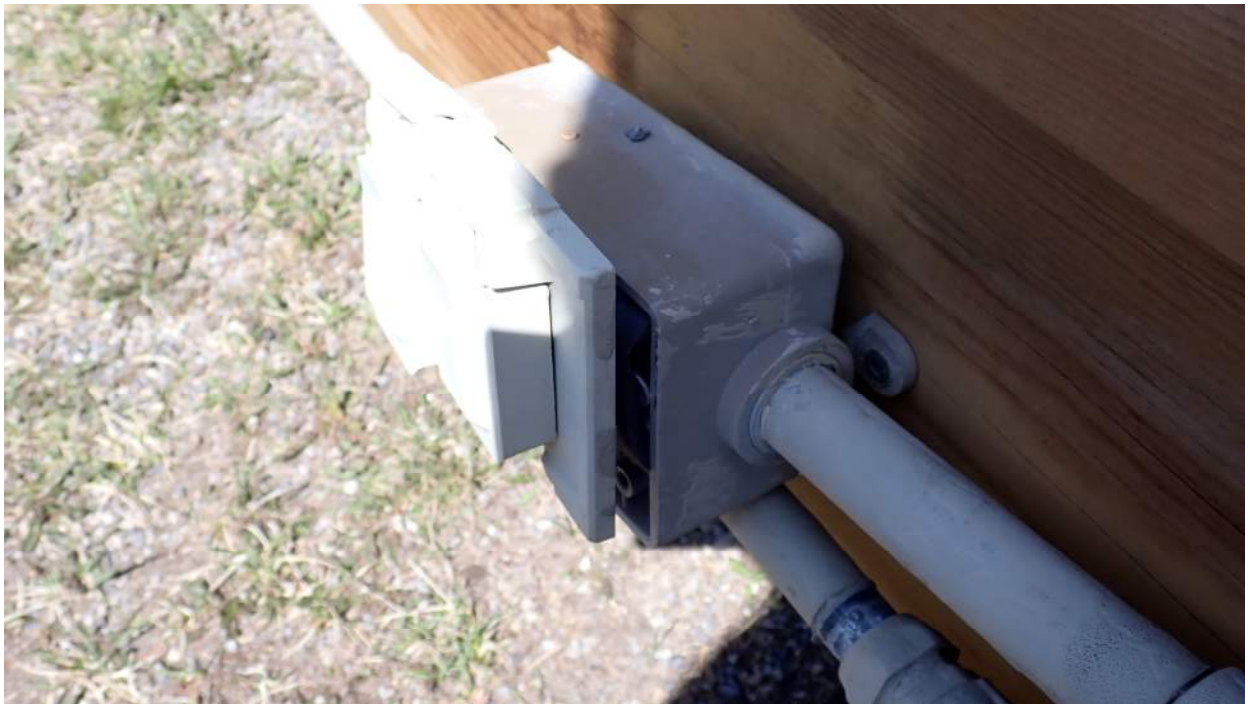
Photo 10 Parking Stall Receptacle Requiring Repair
