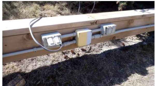
Parking Stall Receptacles
