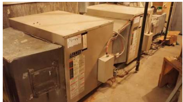
Corridor Make-Up Air Unit
