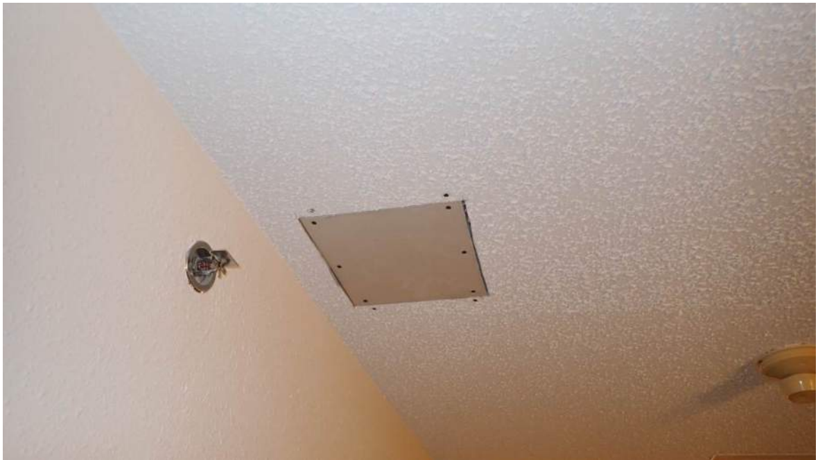
Photo 8 Localized Corridor Ceiling Damage Requiring Repair
